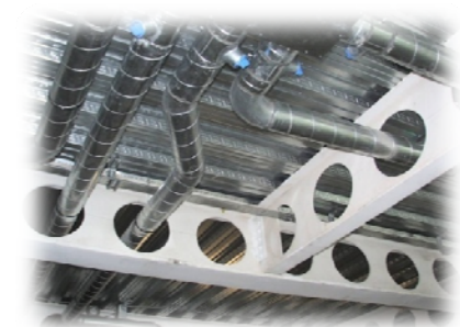
Figure 10: Cellular Beam System Integrating Mechanical Equipment Photo courtesy of CMC Steel Products
